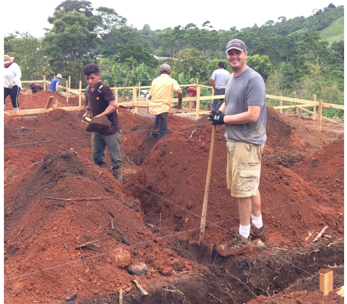
Rosen Hagood attorney Chip Bruorton has traveled to Honduras six times to volunteer with Habitat for Humanity to build homes on a parcel of land purchased by Bruorton’s church.
